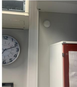
Motion sensor placed high to indicate room activity.
