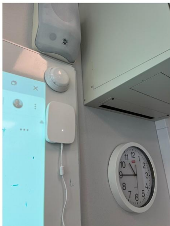
Cloud Connector and motion sensor installed near the board.
