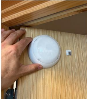
Motion sensor and temperature sensor mounted in a room.
